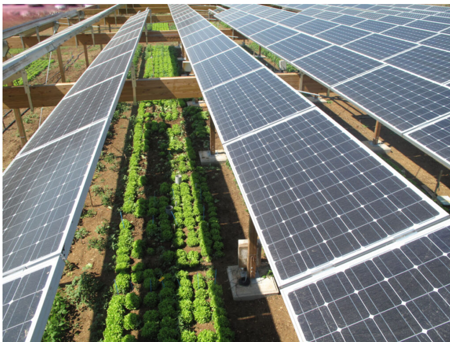
FIGURE II.1 – Installation expérimentale de Montpellier. ©Dupraz
