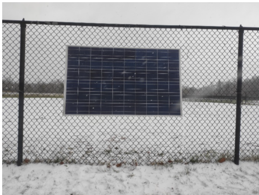
FIGURE II.4 – Installation low-cost sur barrière existante. ©S. Masna et al.
