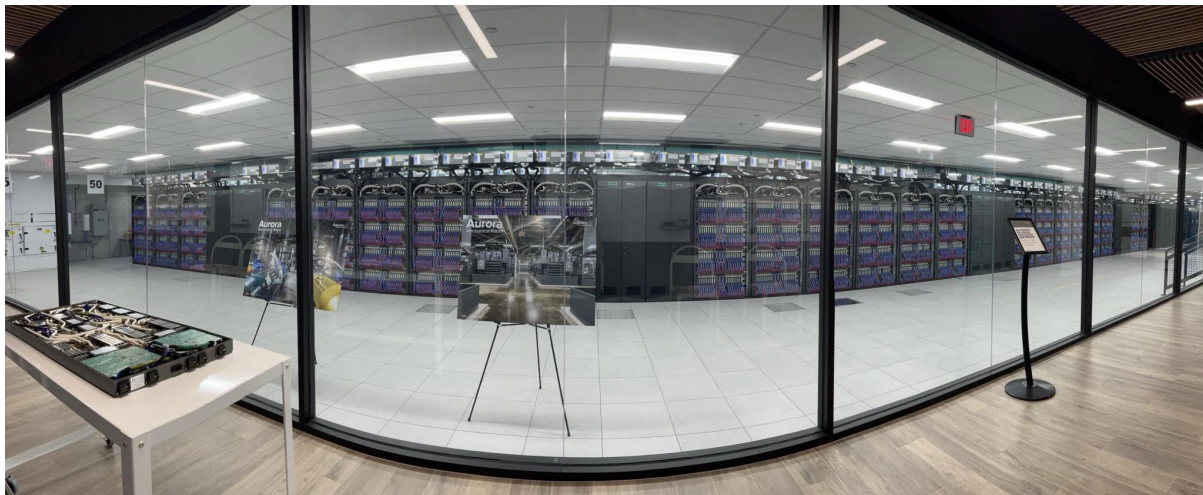
Figure 1.1: Picture of the Aurora supercomputer at Argonne National Laboratory, taken by me. Only the first row of racks are visible, there are 7 more rows hidden behind it. You can see one computing blade equipped with 2 processors and 6 accelerator (Intel GPU) on the bottom left, there are 10624 blades in total on the supercomputer.
