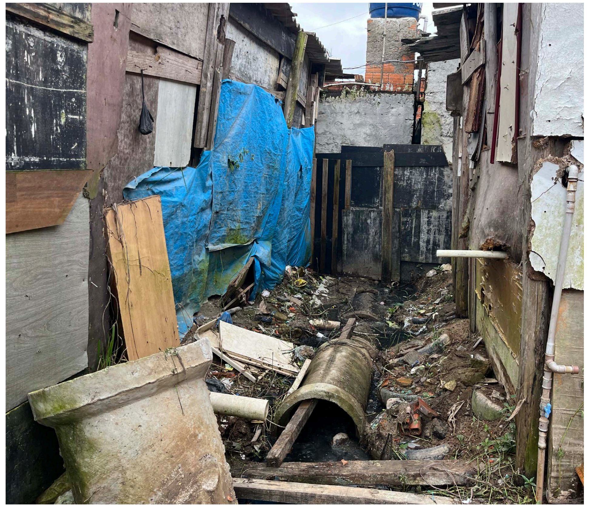
Open sewer clogged with garbage
