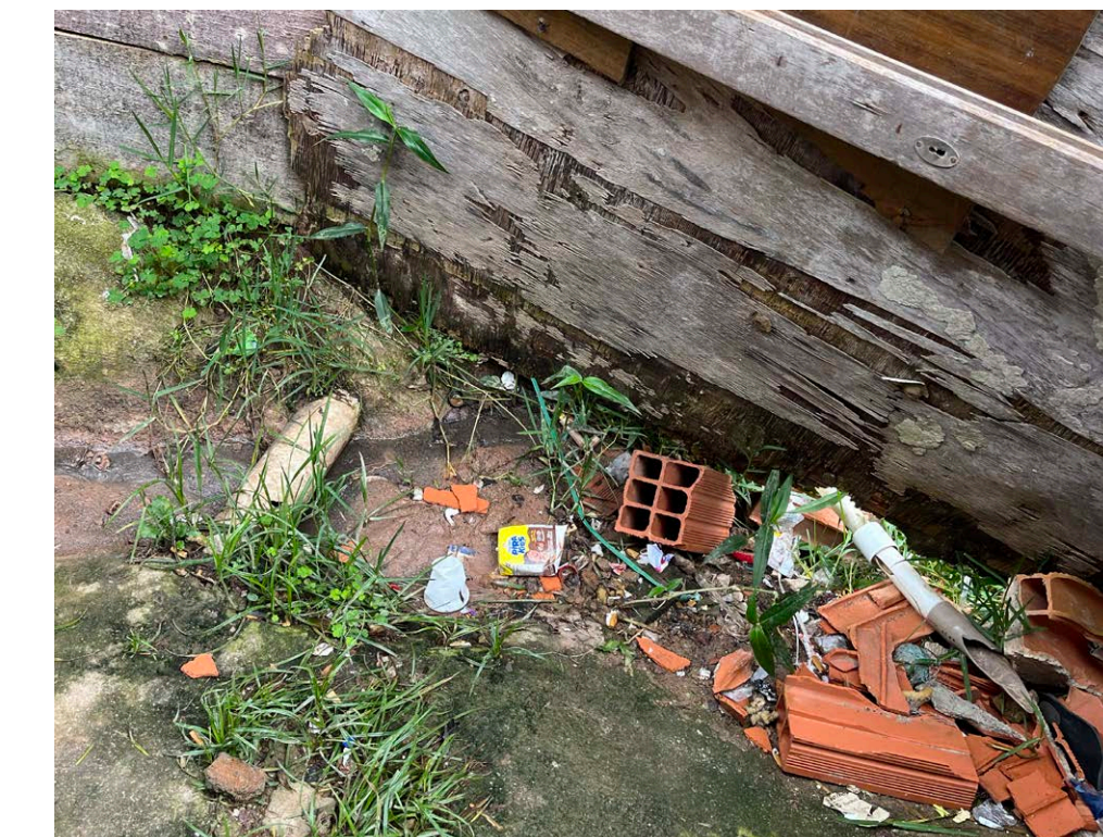
Sewer clogged with garbage
