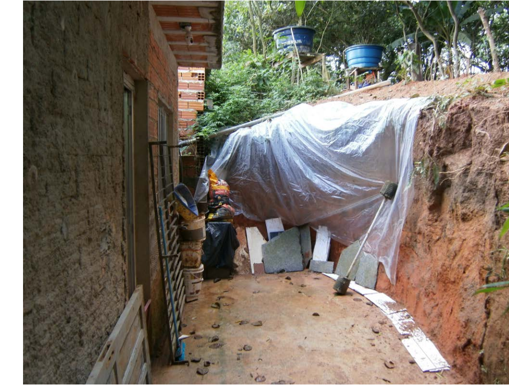
Collapsed embankment covered with a protective tarp
