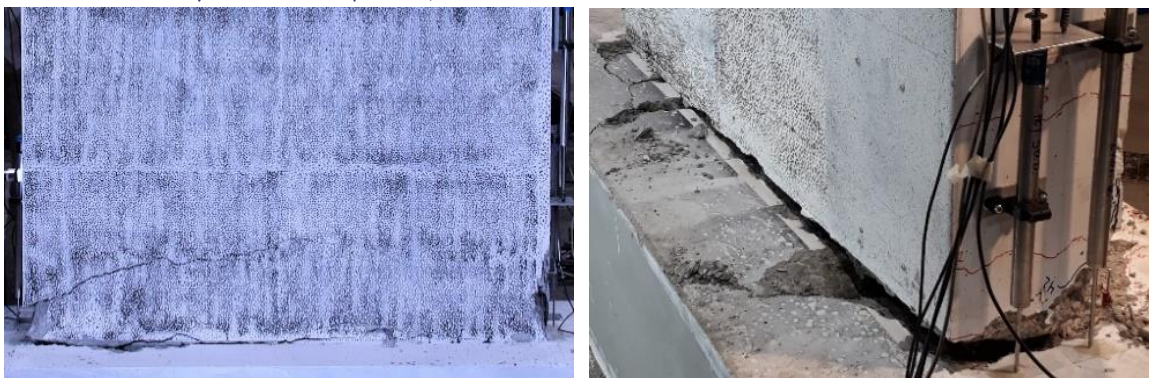
Figure 18 Close-ups on the base of both units: at the end of the test (LS47) for RC wall (right), and the failure (LS51) for RC+SMA wall that occurred at 0.9% (left).
