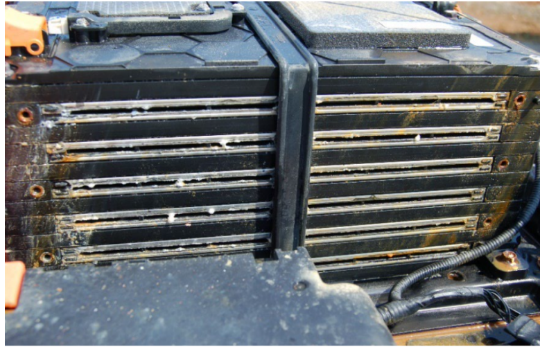
Figure 4.5: Degradation of the battery cells and module
