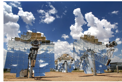
Figure 2.4: A parabolic dish system installation, from http://www.aveva.com/EN/solar-220/aveva-solar.html .
