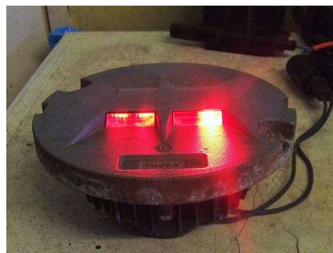
Figure 1.4: Ground directional lights installed at holding points, on the taxiway. [2]
