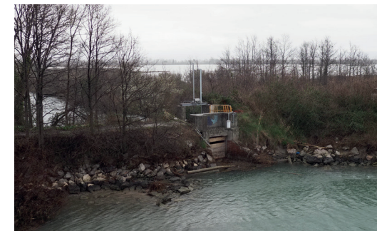
Fig. 38 Sluice broken during a storm
